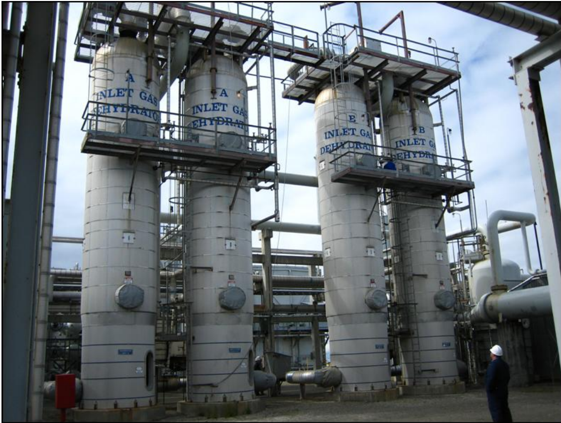
Figure 1: Kenai LNG Facility Dehydrators
