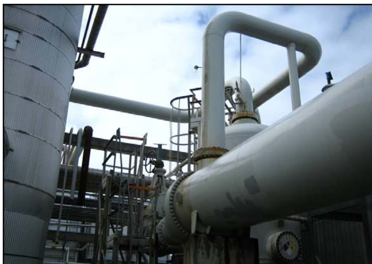
Figure 4: Kenai Gas to Gas Exchanger (Dehydrator Inlet Chiller)
